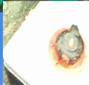
Bad install examples
